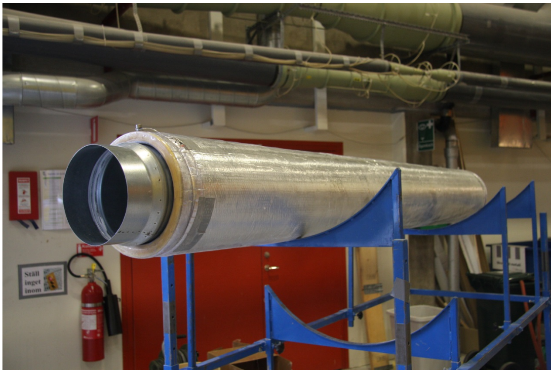
Picture 3 - pipe connection with diameter of 200 mm.
